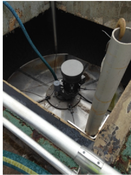
New Mixer on Reactor 1
