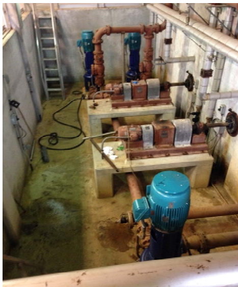
New Grit Pumps
