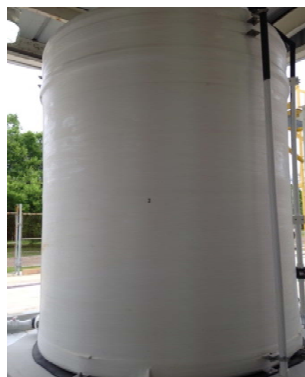
New Sodium Hypochlorite Storage Tank
