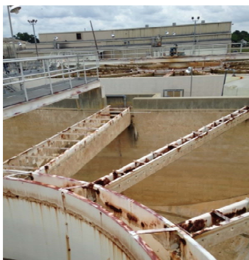
Corrosion on Clarifier Troughs
