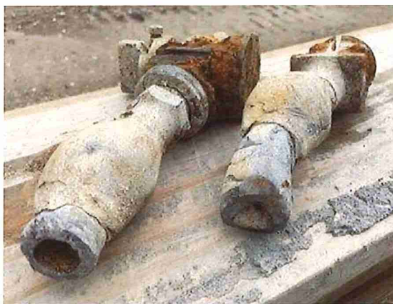
Portions of lead service line removed from residential street in New Orleans
