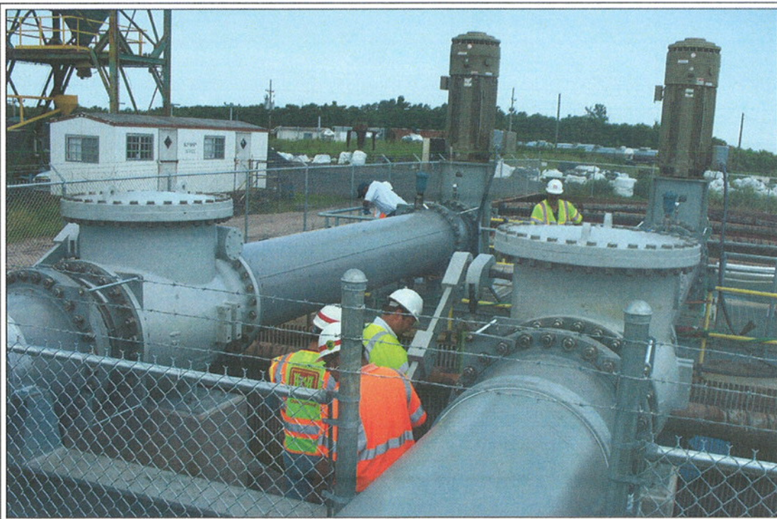
The Elaine Street Drainage Pumping Station in Eastern New Orleans, destroyed by Katrina's floods, has been completely restored by the U.S. Army Corps of Engineers. The $3.2 million project included the installation of 2 new vertical pumps, motors and all new controls and supporting instrumentations. The station was the last to be completed as part of a $39.6 million program whereby the Corps repaired 23 hurricane-damaged drainage stations throughout the City.
