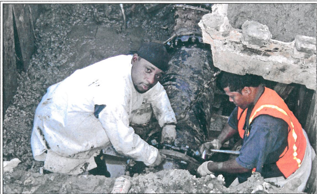
Employees of the S&WB Networks Division are on duty 24 hours a day for emergencies and scheduled repairs. Here, two members of a crew repair a sewer line deep below the street. In 2007: 1,784 broken sewer mains and sewer house connections were repaired and 1.3 million feet of sewer lines and 9,486 sewer manholes were inspected. Also, smoke inspection of 800,000 feet of sewer lines and television inspection of 173,000 feet were completed. 789 new sewer service connections were installed for homes and businesses.
