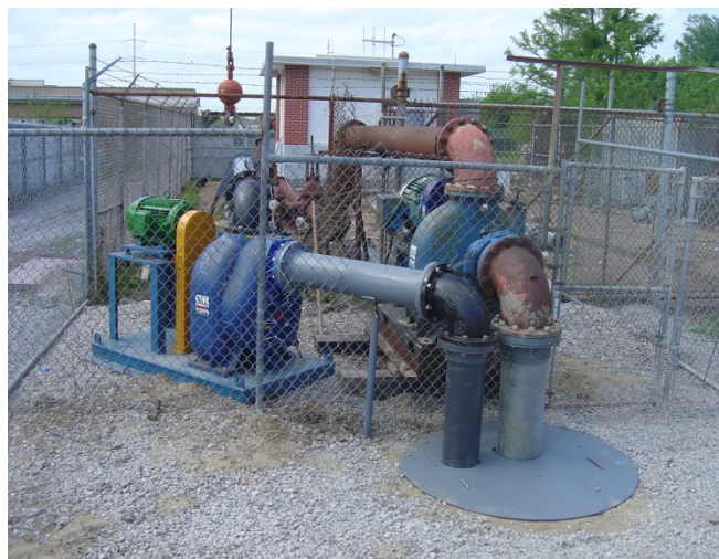
Figure 4 Gorman-Rupp Self Priming Centrifugal Pumps at Blvd X Station
