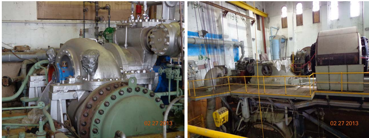
Steam Driven Water Distribution Pump A Turbine 4 Rehabilitation
